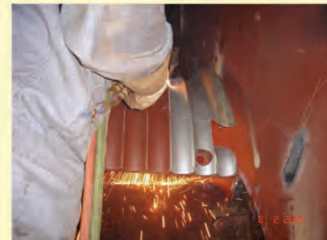
新衬套被焊接到老卷筒上。 The new sleeve is welded onto the old drum.
