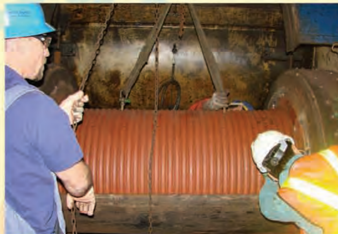
安装Lebus绳槽后,老卷筒焕然一新。 Fitting a Lebus sleeve onto an old drum to make it as good as new.
